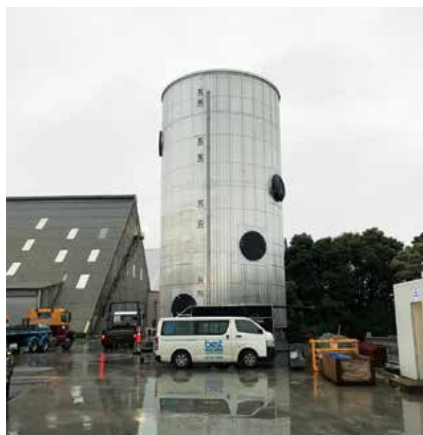
The Mount site's new SO 2 convertor, ready to be lifted into place.
